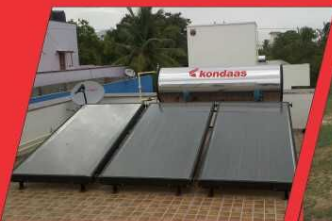
Solar Water Heater
