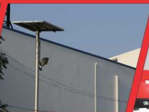
Solar Street Lights
